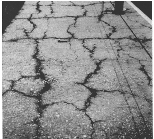
Figure 2-6. Pattern cracking resulting from alkali-silica reaction
