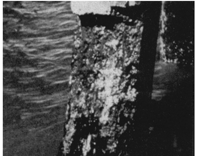
Figure 2-13. Disintegration of concrete caused by exposure to acidic water
