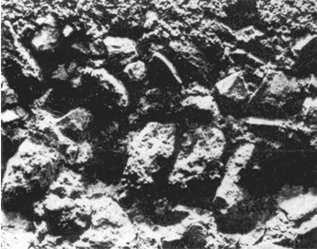
Figure 2-21. Rough, pitted concrete surface caused by cavitation
