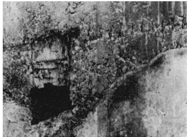
Figure 2-2. Honeycombing and cold joint
