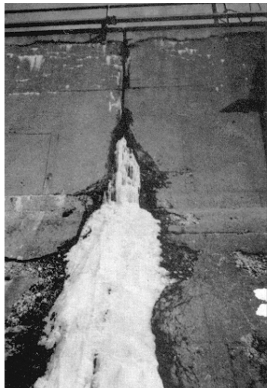
Figure 2-28. Water seepage through joint
