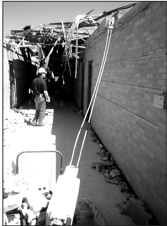
Figure 6-5. Failure in this load path occurred between the bond beam and the top of the unreinforced masonry wall. This school building was in the path of an F4 tornado vortex.
