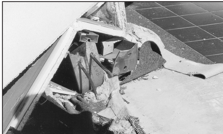
Figure 6-6. These two steel columns failed at their connection to the foundation. The anchor bolts that secured the column released from the concrete (embedment failure) while the anchor bolts that secured the column on the right experienced a ductile failure.
