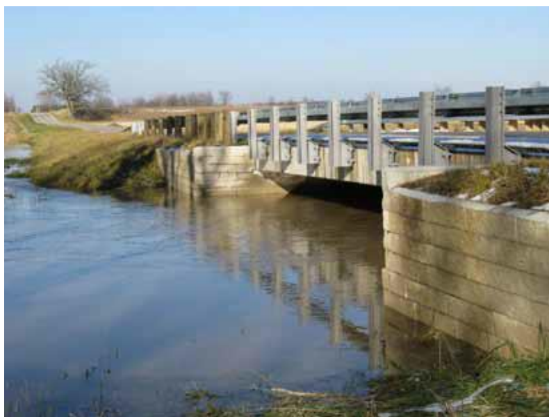
Figure 19. Glenburg Road Bridge under flood conditions.
