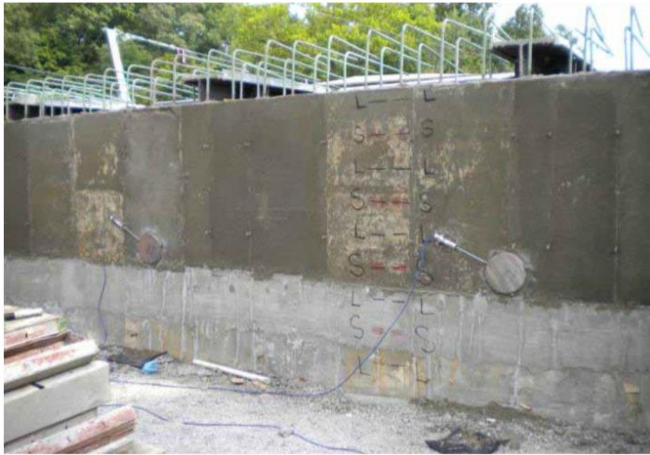
Figure 39. Pressure cells behind back wall on Tiffin River Bridge.
