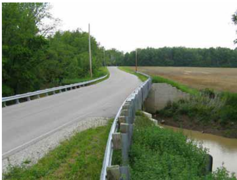
Figure 23. Bowman Road Bridge after 4.5 years.
