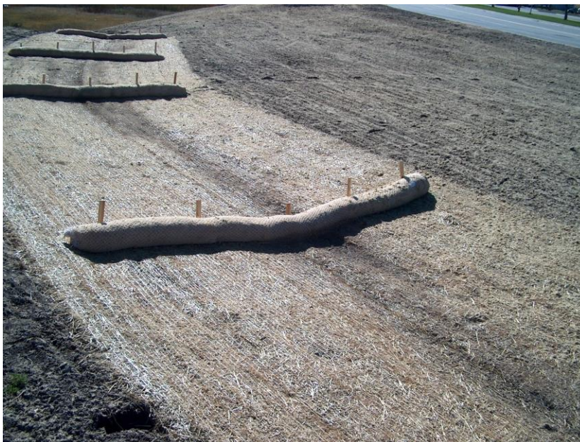
Figure 10 – Erosion Control Blanket
