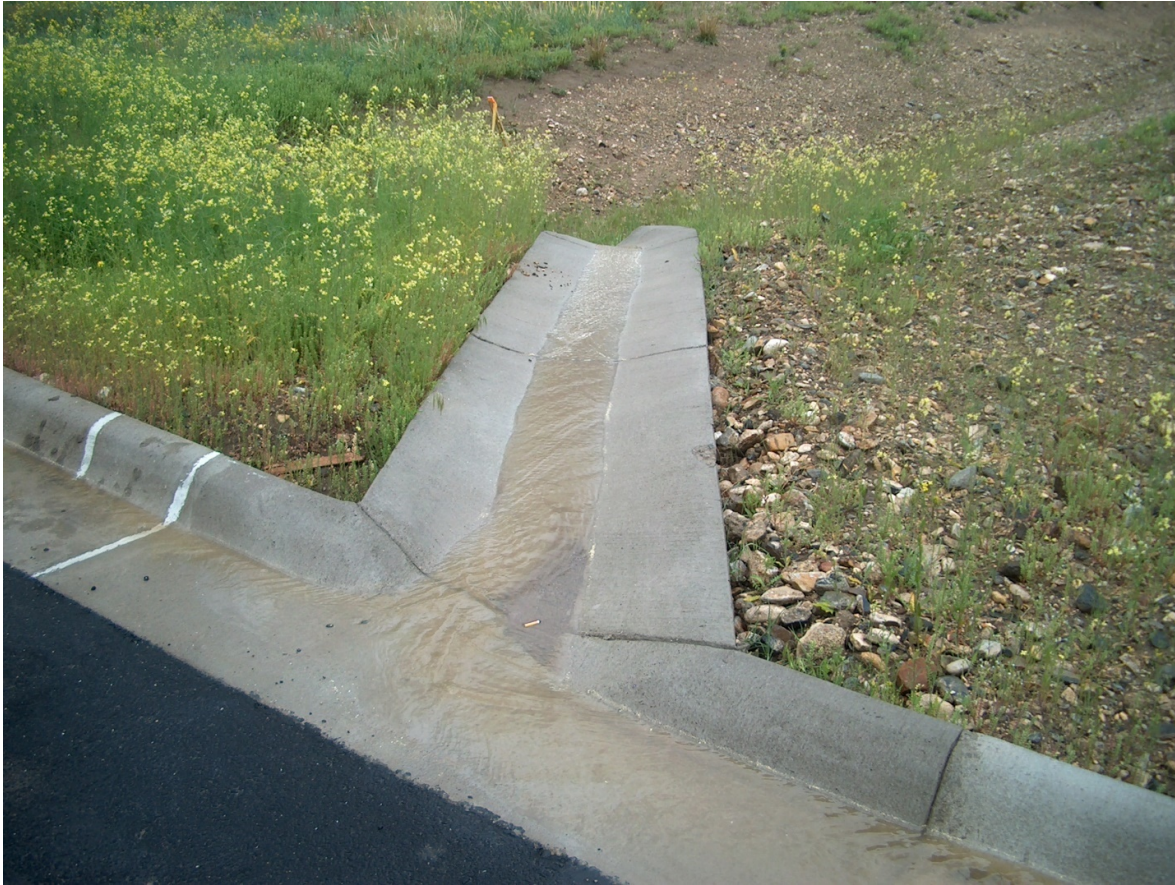
Figure 11 – Curb opening into LID feature
