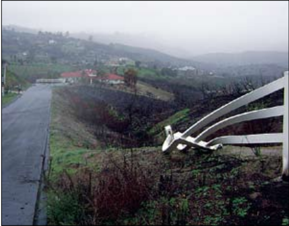
Figure 2. Plastic fences can melt even under moderate wildfire temperatures (FEMA field team).
