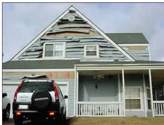
Figure 1. Vinyl siding that melted and warped during a wildfire (firecenter.berkeley.edu).
